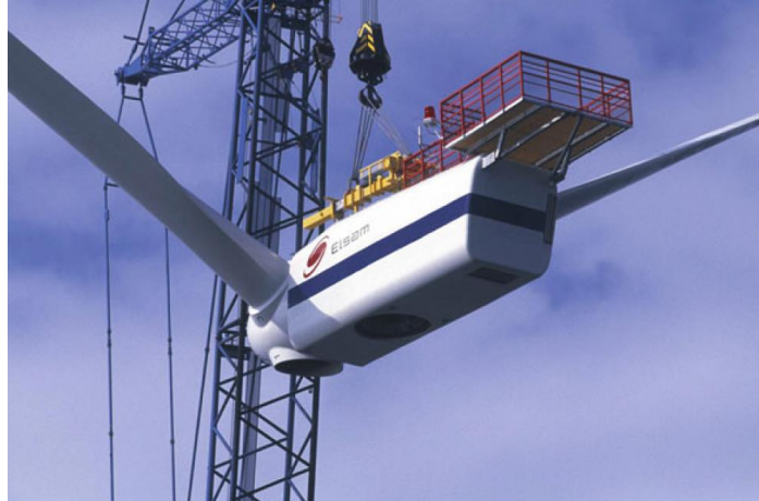
Fig 5. Lifting the pre-assembled nacelle, rotor hub, and two blades as bunny ear configuration [22] 1
