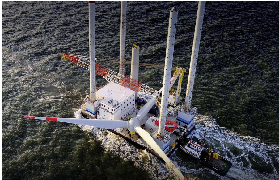
Fig. 8. Jack-up barge J-114 applied for the installation of Alpha Ventus and Belwind windfarms 1
