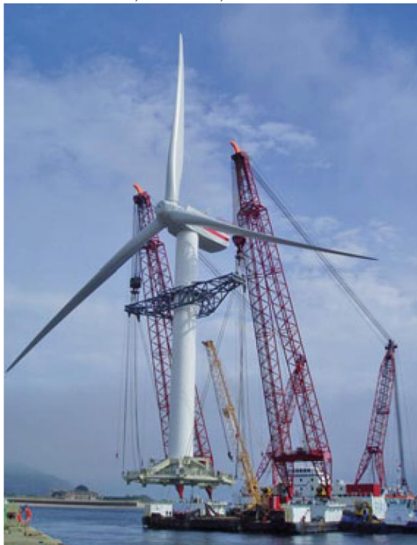
Fig. 6. Lifting the whole WT in a single lift at Beatrice wind farm [22] 2
