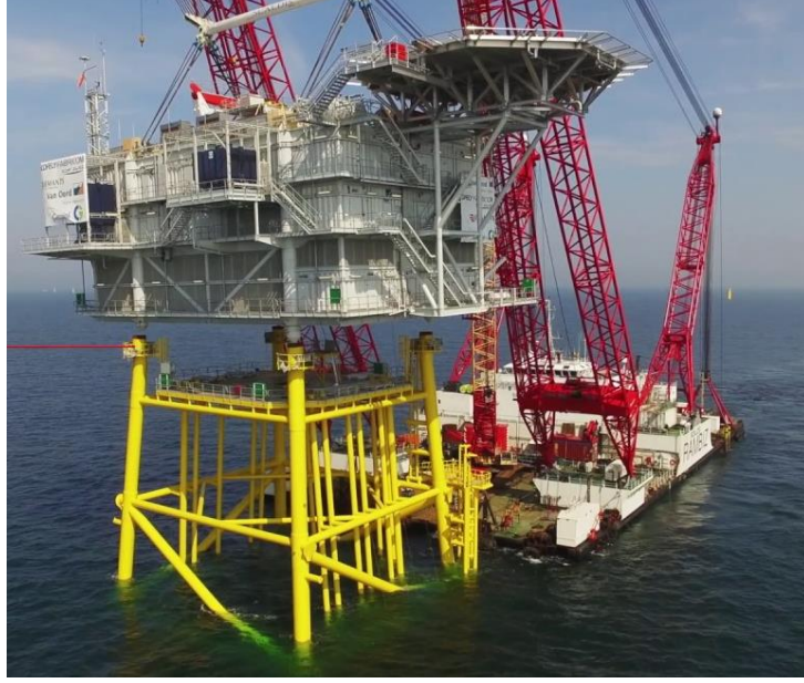
Fig. 31. Installation of the topside of the OS in Gemini offshore wind farm in the Netherland 1
