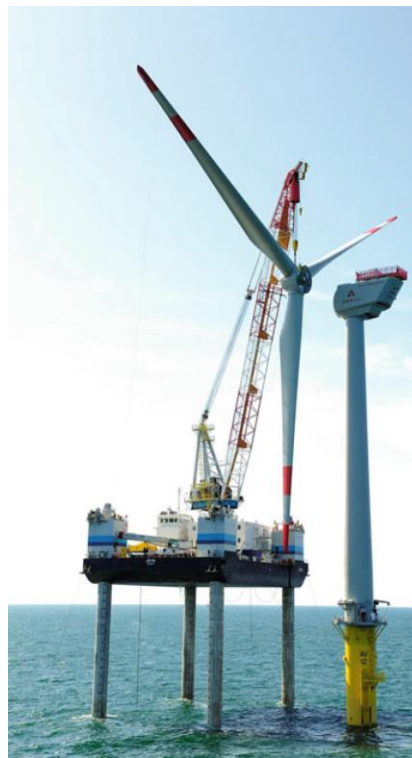
Fig. 4. Installation of the pre-assembled rotor hub and blades in a single lift at Alpha wind farm [22] 2
