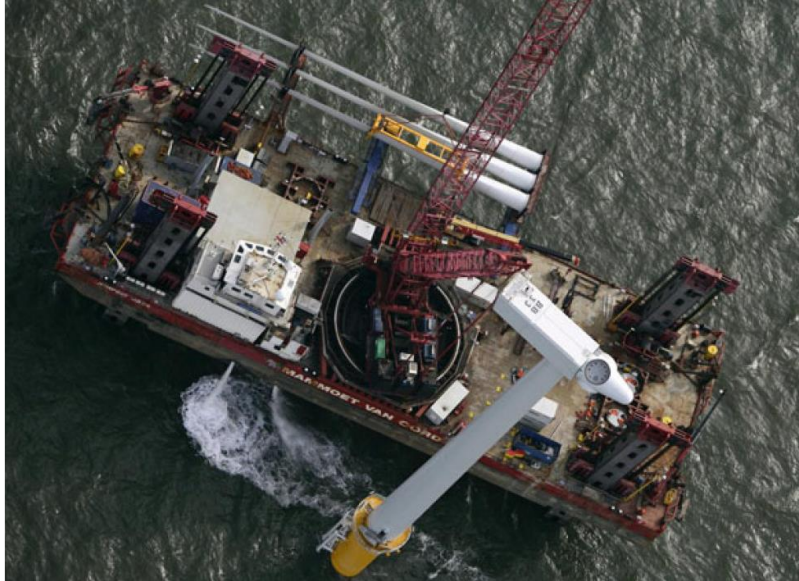
Fig. 3. Installation of nacelle and hub in a single lift at Burbo Bank, Siemens [22] 1
