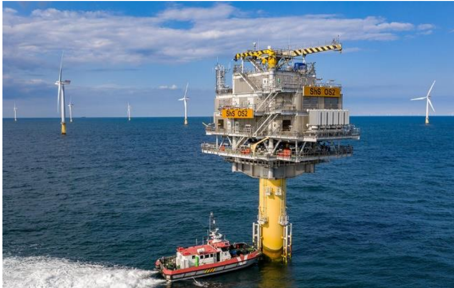
Fig. 7. OS with monopile foundation in Sheringham Shoal OWF, England 1
